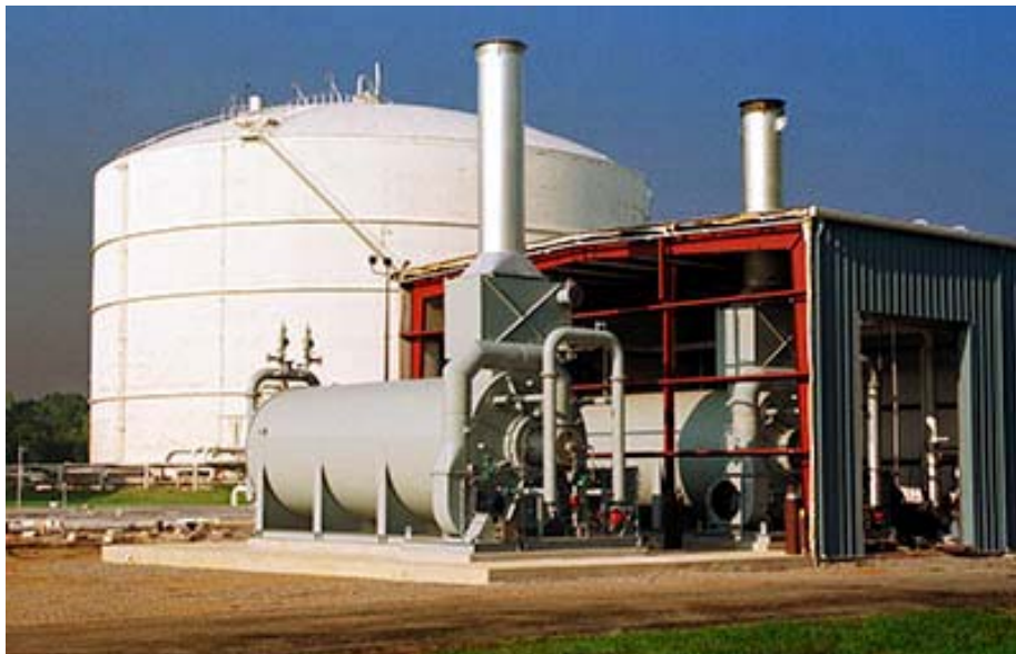
Figure 6: Redundant gas-fired package heaters supporting small G/W vaporizer installation
