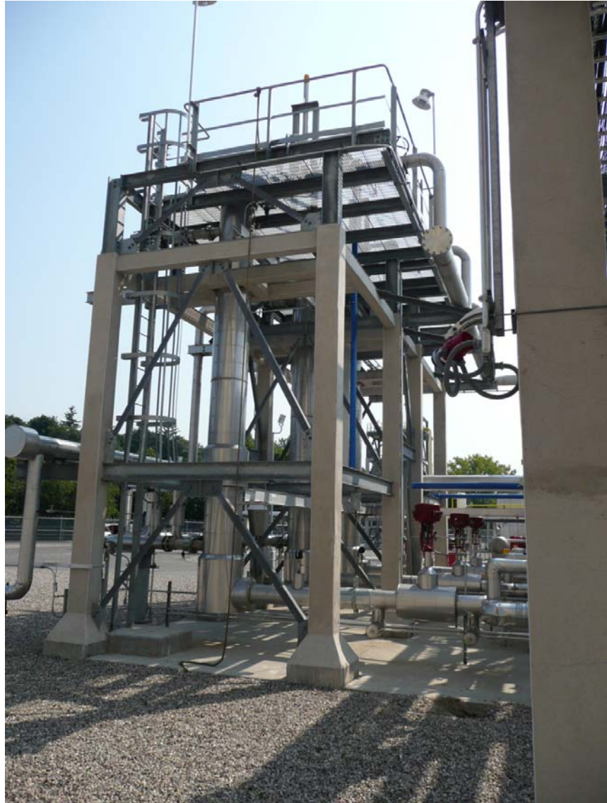
Figure 5: 3 x 30 mmscf Each Shell & Tube LNG Vaporizer Installation
