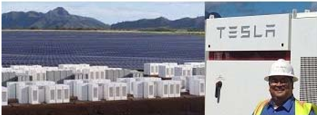
Figure 14-1. KUIIC Tesla Solar Power Plant (left). GPA AGMETS tours facility (right) (2017)
